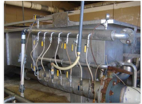
Figure 1 Original DAFs unable to treat water
