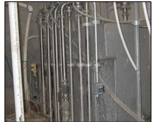
GEM System with Liquid Gas Mixing Heads that manage the flocculation process.
